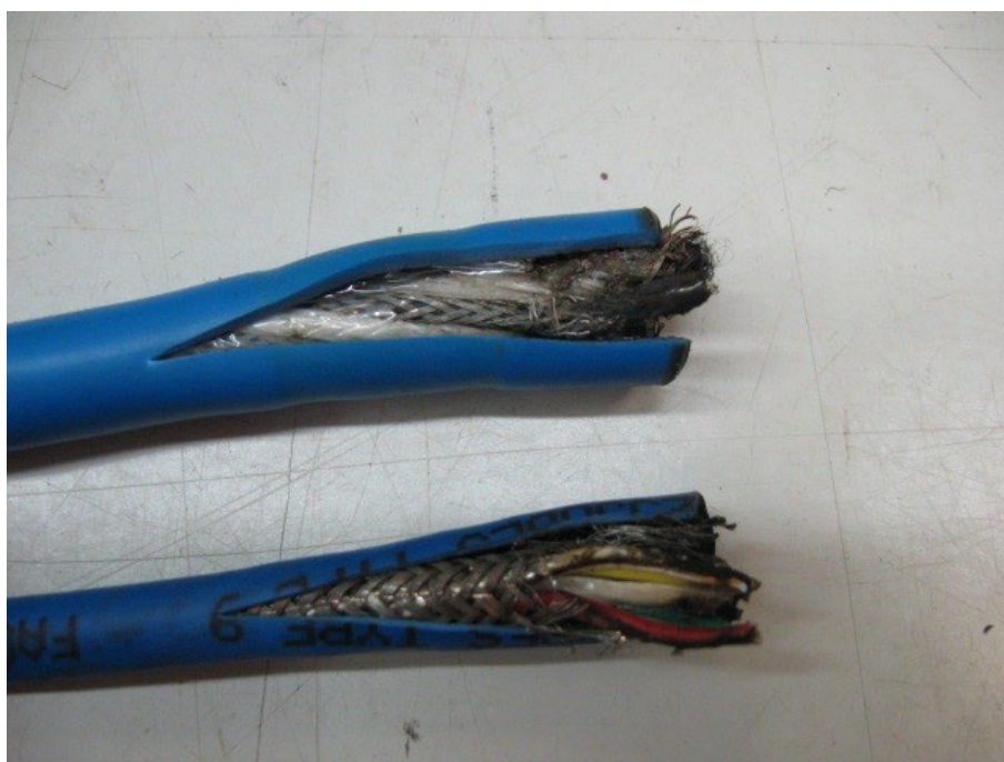
Figure 3 – Testsafe 2016 – Damage to the exposed cable end, but with no flame transmission
